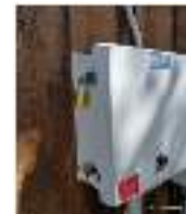
New Pump Control
